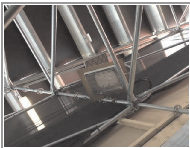
Fig. 5. Access point with external antenna directed upwards under the seats in the hockey venue.
