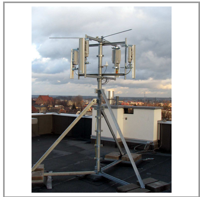
Fig. 1. One of INEA's WiMAX base station.
