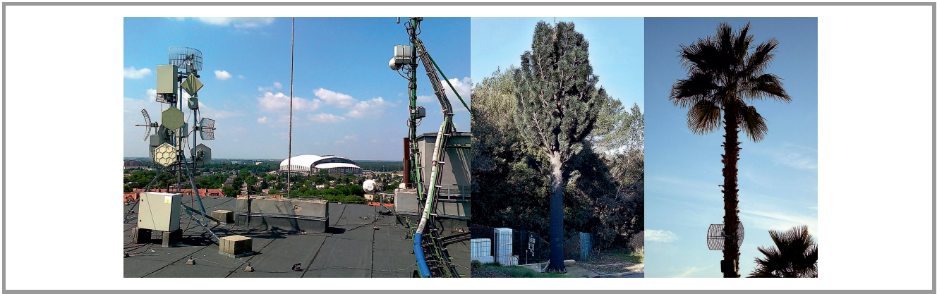
Fig. 1. A rooftop cellular and IEEE 802.11 networks base station (left) (Poznań, Poland, July 2011), an artificial tree used as a base station on a hillside (middle) (Sophia Antipolis, France, March 2016), a wireless station on a palm tree (right) (Athens, Greece, October 2013).
